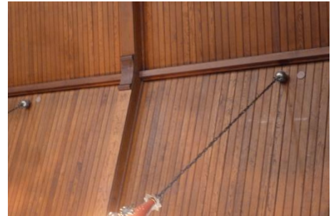
It's difficult to locate the sprinklers.
