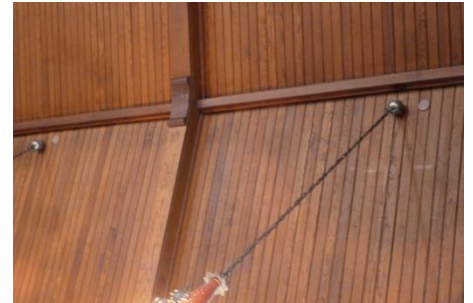
It's difficult to locate the sprinklers.
