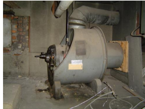
the electric motor and pump
